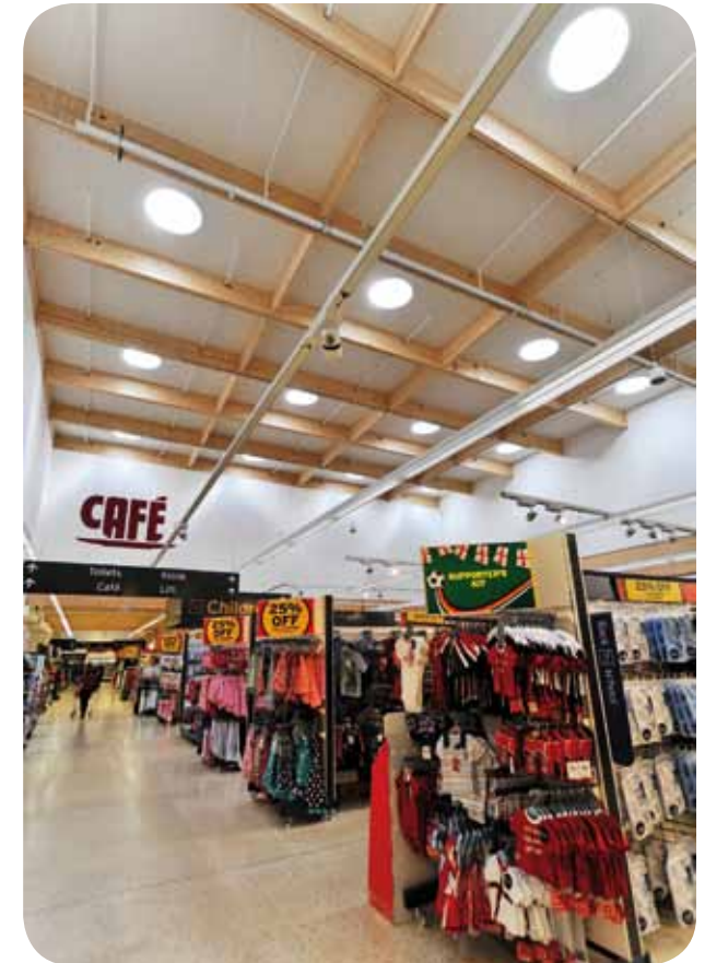
Sainsbury's, Durham - 1000mm diameter SUNPIPE natural daylight systems were used to light the double height sales area
